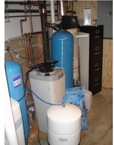
Old Iron Filter
