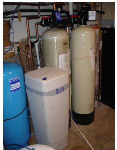
New Iron Filter System
