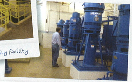
Water pumps providing Maple Grove's clean water.
