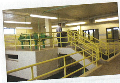
Control Panel at Maple Grove utility facility.
